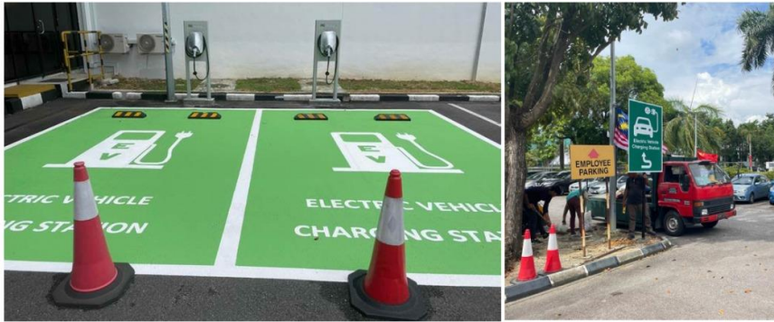
Figure 1: Free EV charging facilities installed for employees and visitors
