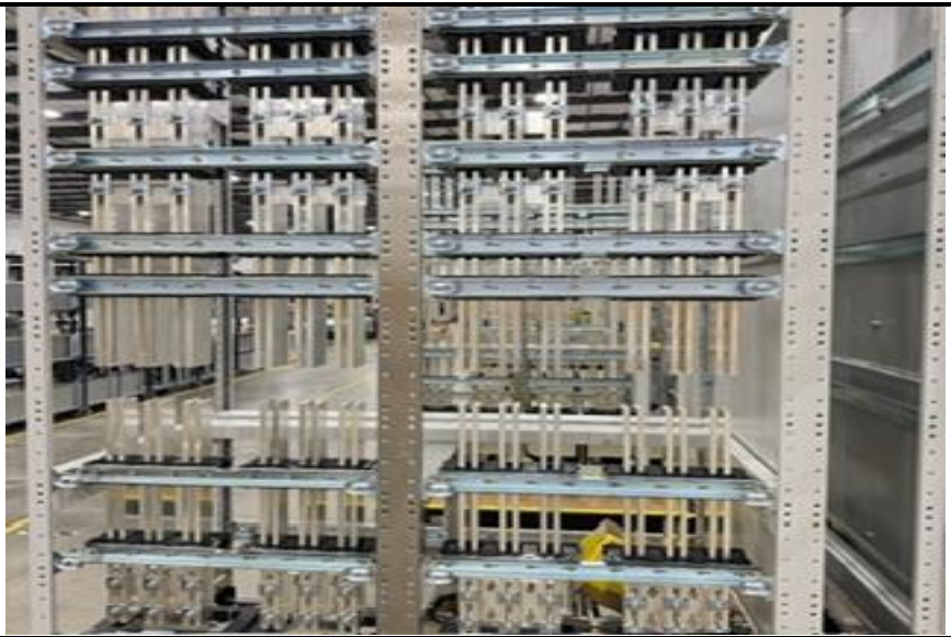
Fig 7: Copper rods used in racks
