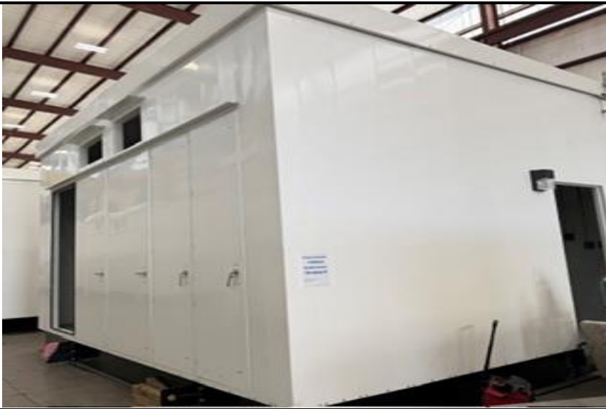
Fig 3: Electrical room for data centre
