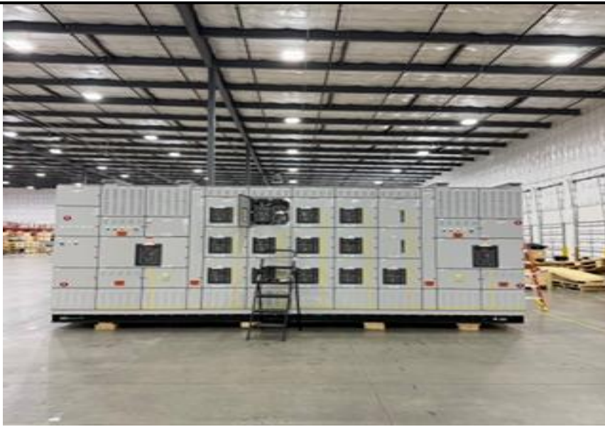
Fig 5: Equipment to be installed in electrical rooms
